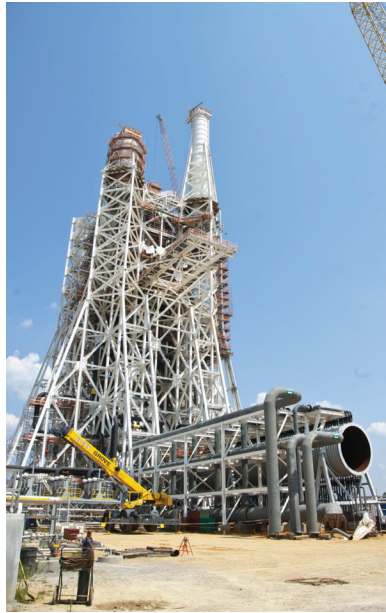
Photo 2: The A-3 Test Stand is the first large test structure to be built at Stennis Space Center since the 1960s.
