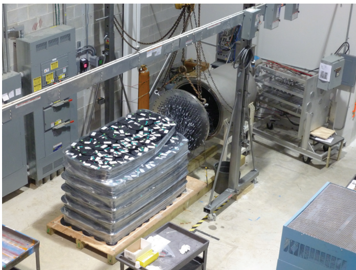
Photo 4: With several hundred feet of cable run, each feedthrough is prewired and tested prior to installation. (Photo courtesy of Douglas Electrical Components.)
